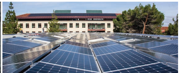
Roof mounted solar array.
