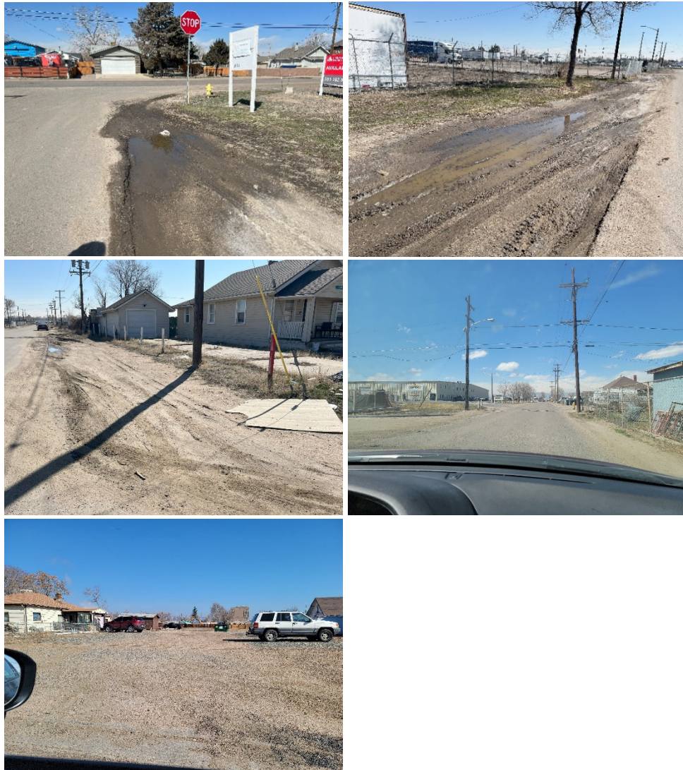
Figure 18. Lack of pavement, curb, sidewalks, lighting, or drainage
