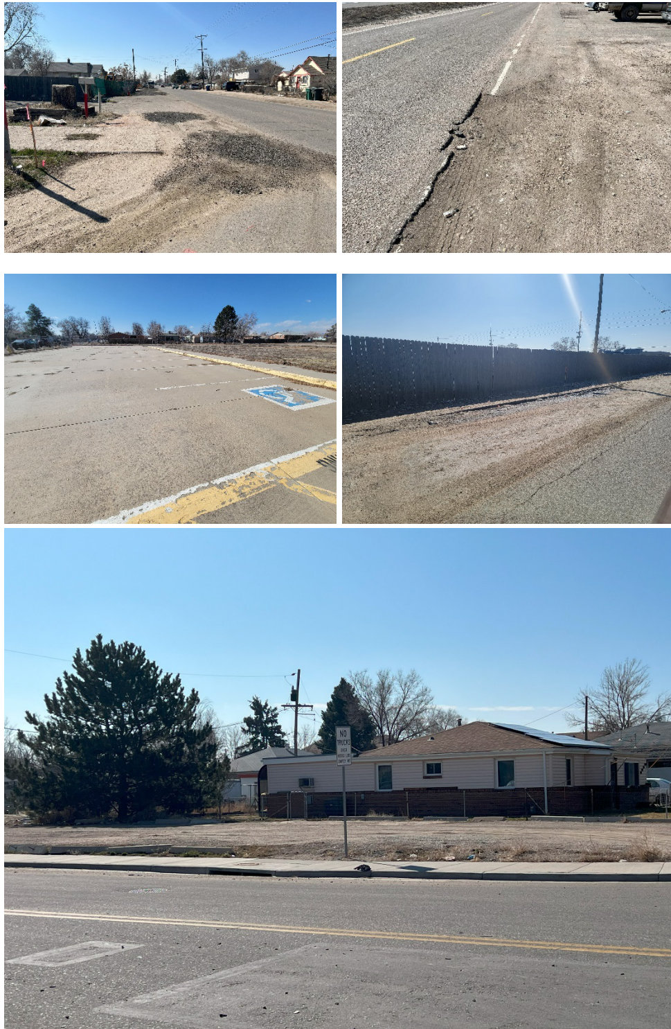
Figure 17. Deteriorated on-site parking surfaces, curb & gutter, or sidewalks
