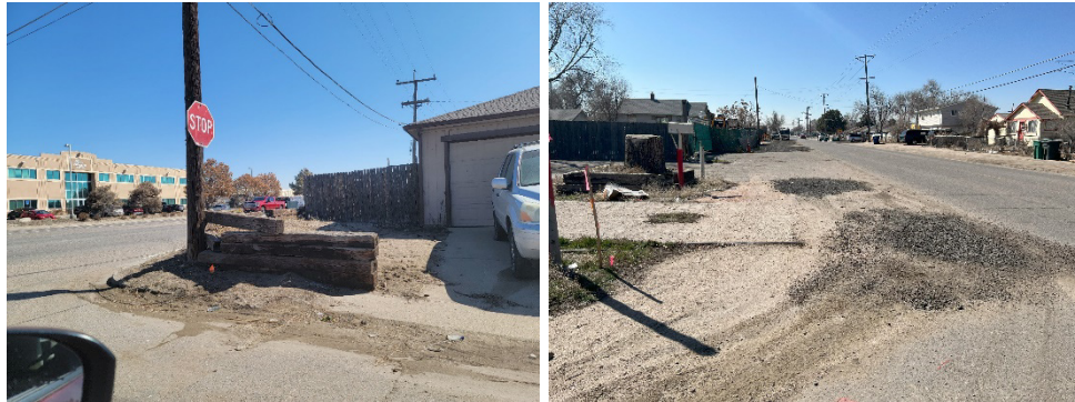
Figure 12. Cracked or uneven surfaces for pedestrians
