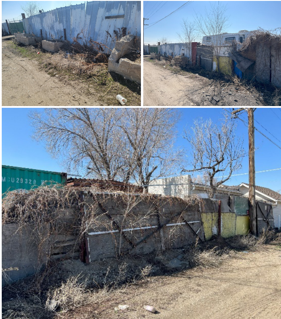
Figure 16. Deteriorated fences, walls, or gates
