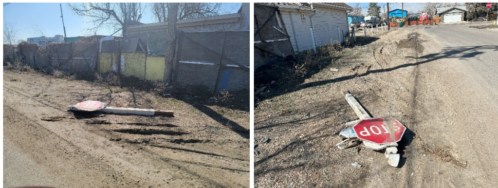
Figure 15. Deteriorated signage or lighting
