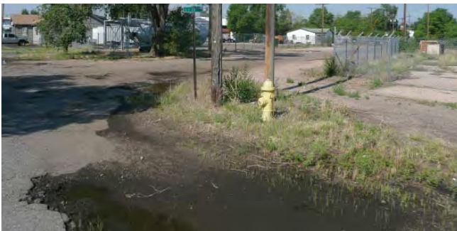
There are many storm drainage issues in the neighborhood
