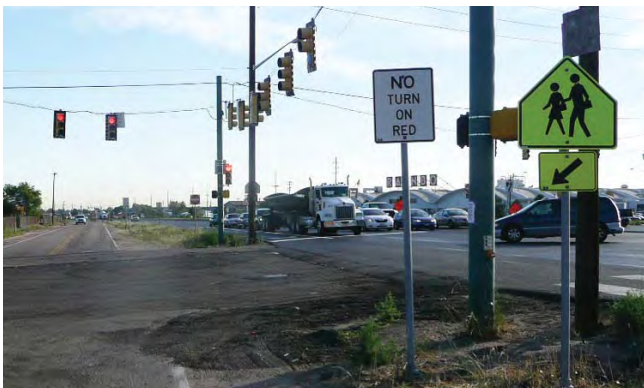
Pedestrian safety must be addressed at 72nd Avenue and Brighton Boulevard
