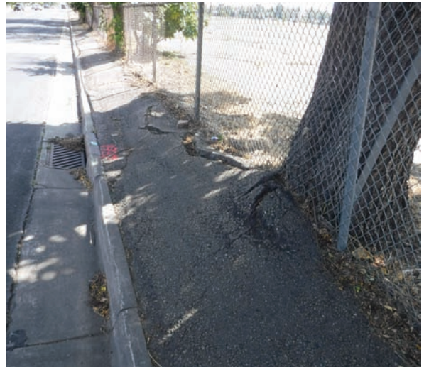
Lack of Sidewalk
