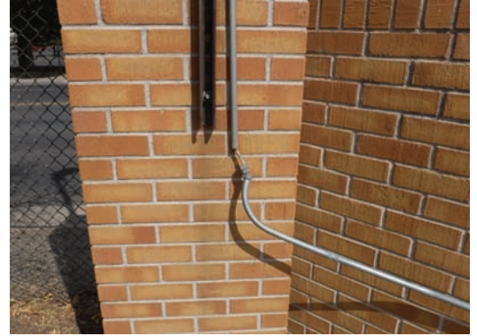
Unsafe/Exposed Electrical Wire
