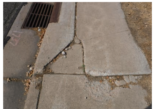
Cracked/Uneven Pedestrian Surfaces
