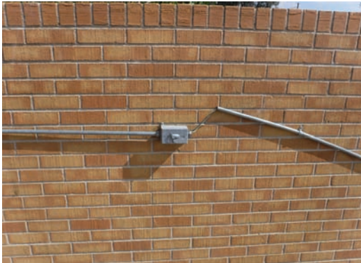
Unsafe/Exposed Electrical Wire
