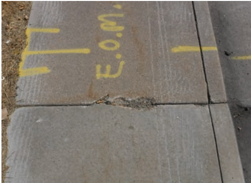
Cracked/Uneven Pedestrian Surfaces
