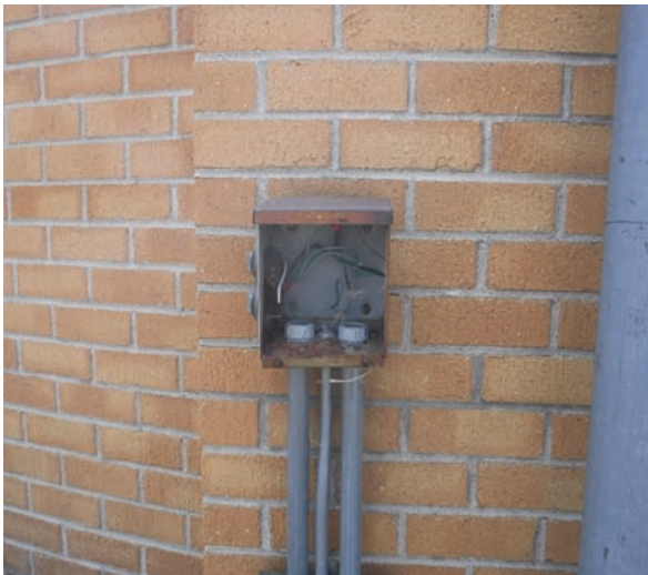
Unsafe/Exposed Electrical Wire
