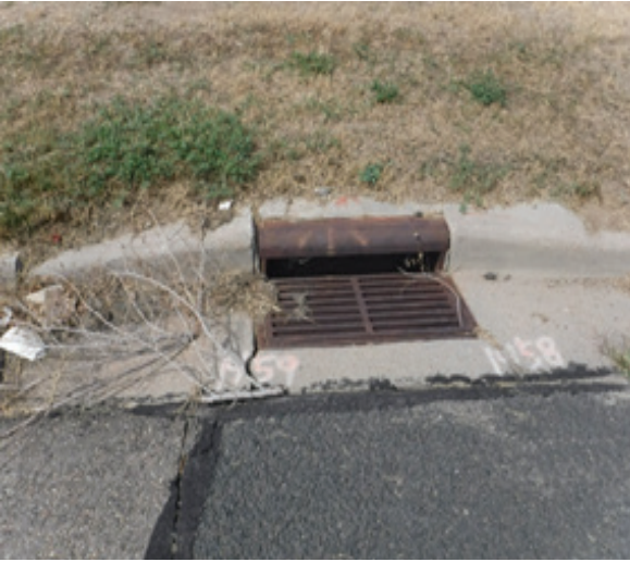
Deteriorated Stormwater Systems
