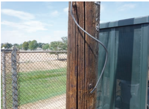
Unsafe/Exposed Electrical Wire
