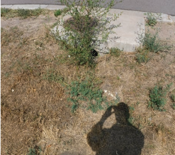
Deteriorated Stormwater Improvements
