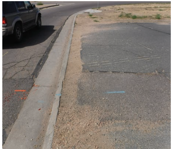
Lack of Access to Dahlia Street right-of-way
