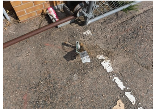
Unsafe/Exposed Electrical Wire
