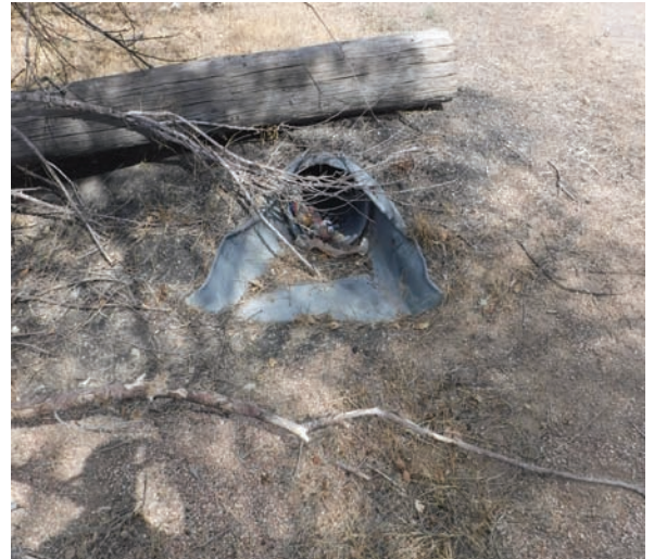
Deteriorated Stormwater Improvements
