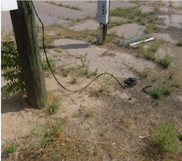
Unsafe/Exposed Electrical Wire
