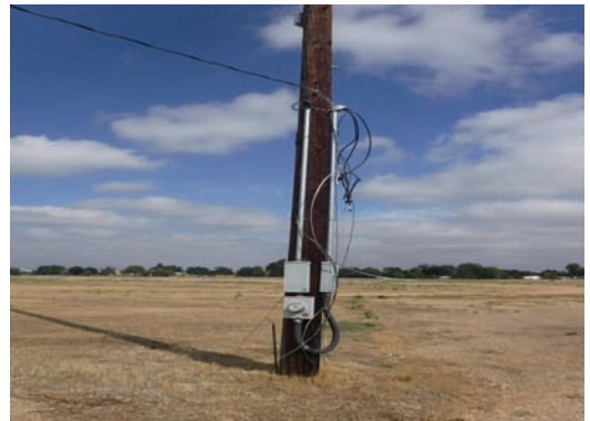
Deteriorated Electrical Pole
