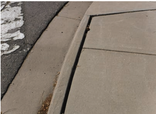
Cracked/Uneven Pedestrian Surfaces
