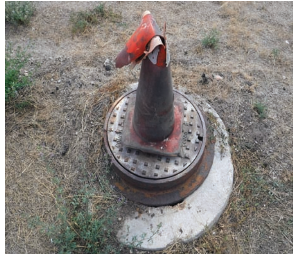
Dilapidated/Deteriorated Accessory Structure
