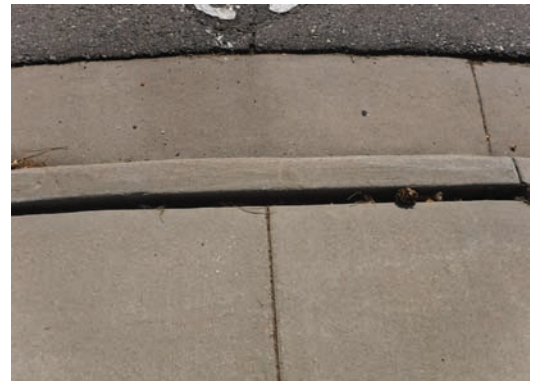
Cracked/Uneven Pedestrian Surfaces
