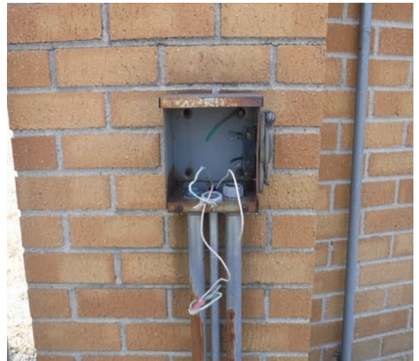
Unsafe/Exposed Electrical Wire
