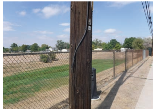
Unsafe/Exposed Electrical Wire
