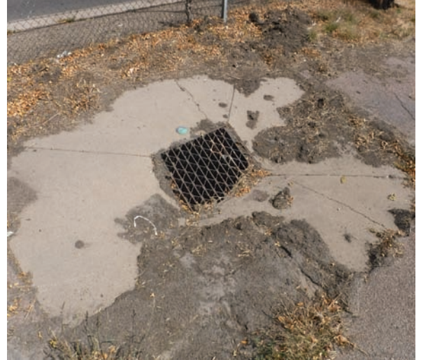
Deteriorated Stormwater Improvements
