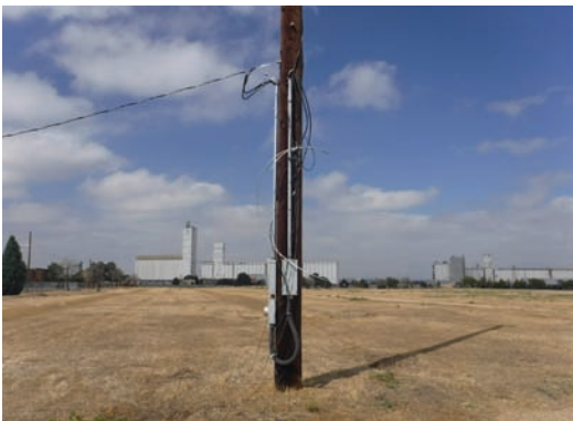
Deteriorated Electrical Pole
