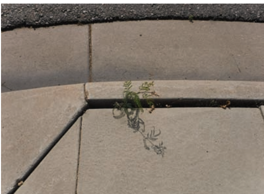
Cracked/Uneven Pedestrian Surfaces
