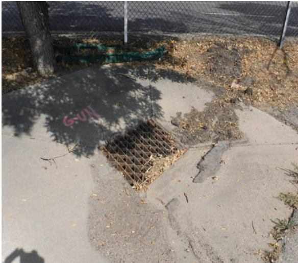
Deteriorated Stormwater Improvements
