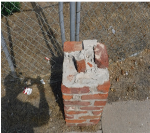
Deteriorated Support Post
