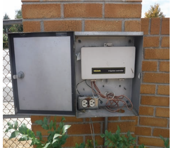
Unsafe/Exposed Electrical Wire
