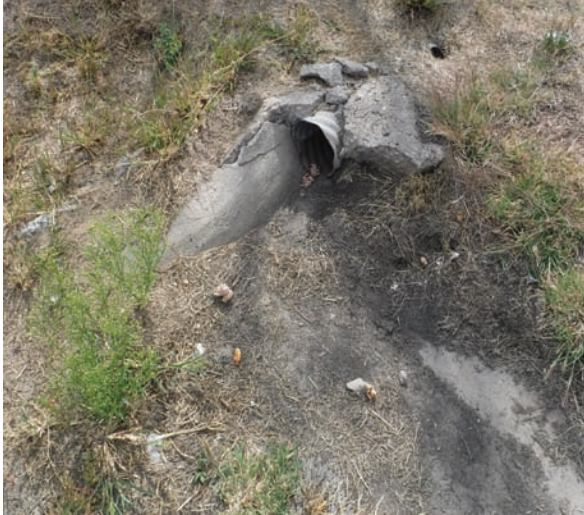
Deteriorated Stormwater Improvements
