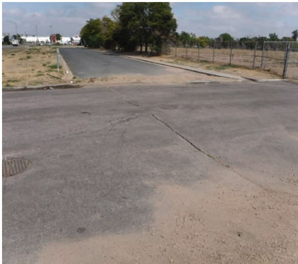
Lack of Access to Dahlia Street right-of-way
