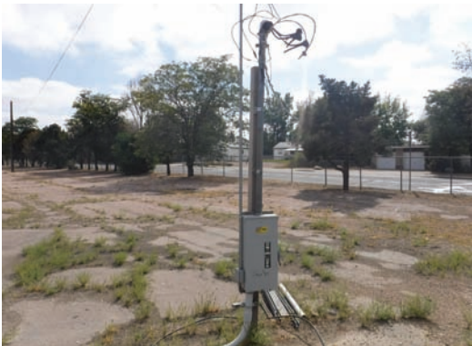
Deteriorated Electrical Pole
