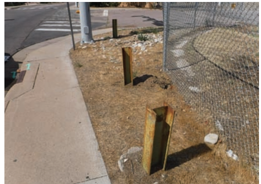
Deteriorated Accessory Structure
