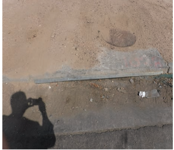
Deteriorated Stormwater Systems
